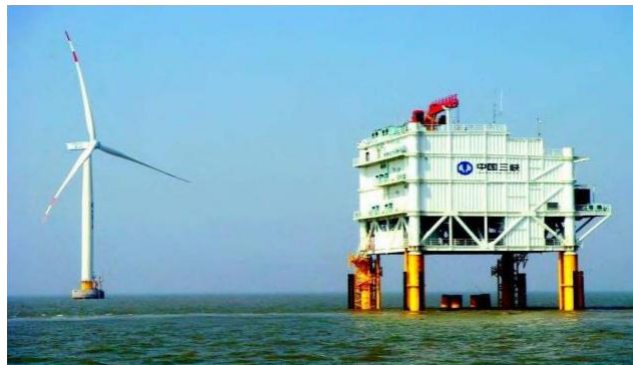
Fig1: Offshore booster station
